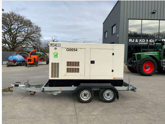
JCB G66QS GENERATOR TWIN AXLE (ST22610)
