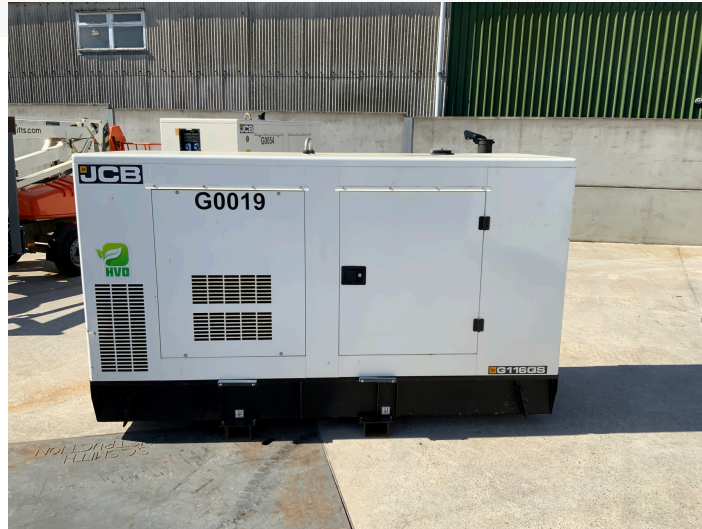
JCB G116QS GENERATOR
